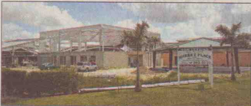
Construction continues at the Naples Big Cypress Market Place. A little smaller than a Wal-Mart, the shopping and entertainment center will include an indoor flea market, winery, entertainment area and convention center.
